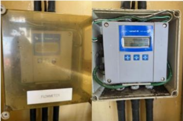
Figure 7: Influent Magnetic Flow Meter Display Unit
