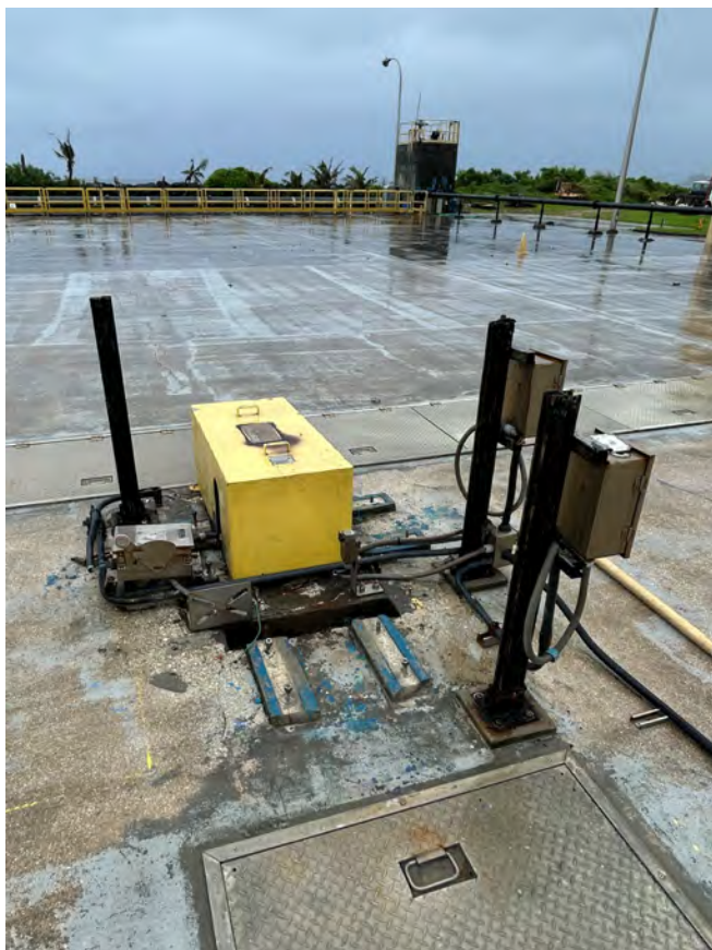
Figure 22: Primary Clarifier Cross Collector 1 (PCCC-2)
