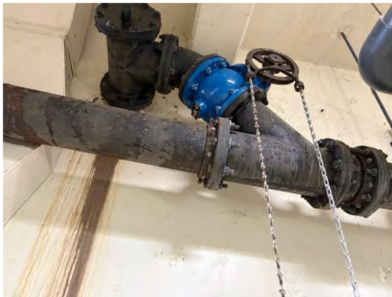
Figure 48: Digester isolation valve (ground floor)
