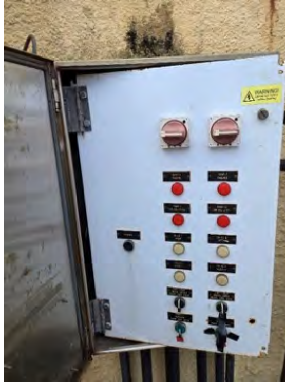
Figure 29: Scum Pump Control Panel
