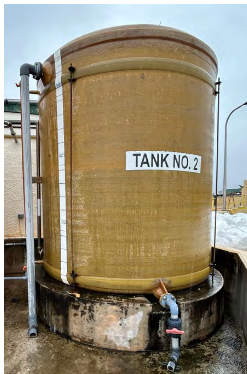
Figure 56: Chemical Day Tank 2 (Tank No. 2)
