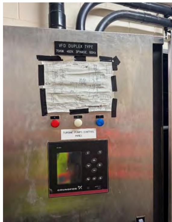
Figure 36: Effluent Pump Control Panel and VFDs
