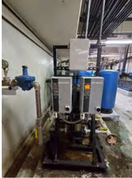
Figure 52: Booster Pump VFDs and Controls
