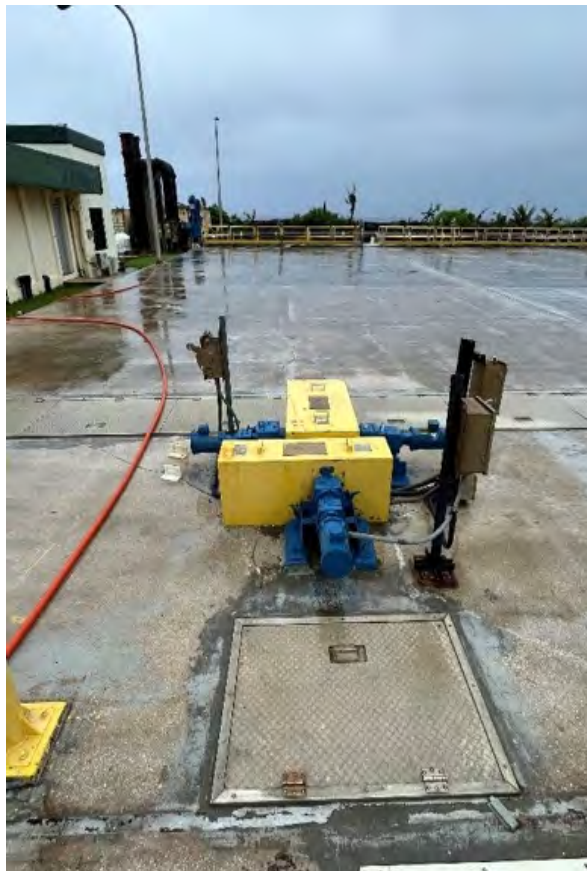
Figure 21: Primary Clarifier Cross Collector 1 (PCCC-1) and Longitudinal Sludge Collectors 1A and 1B
