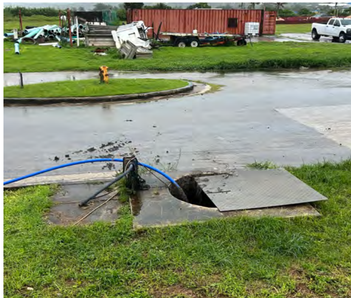
Figure 2: Dewatering Building Sump Pump and Piping
