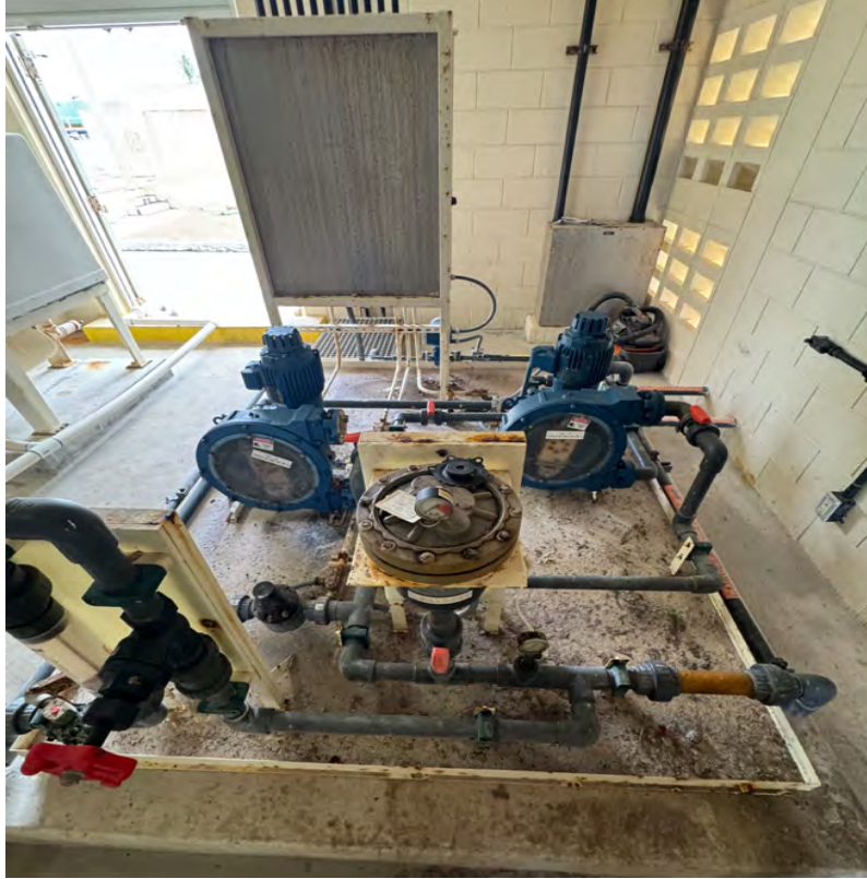
Figure 57: Chemically Enhanced Coagulant Chemical Feed System
