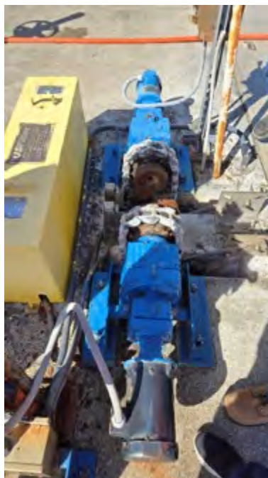
Figure 25: Longitudinal Sludge Collector Clarifier 1 (PC-1A and PC-1B)
