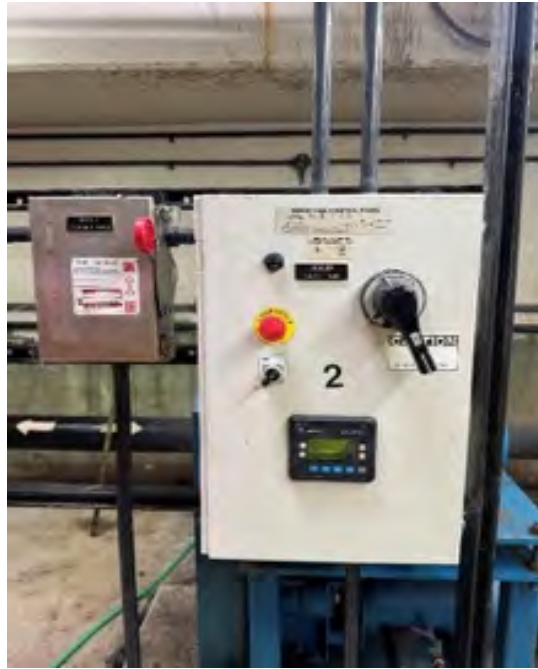
Figure 42: Primary Sludge Grinder and Transfer Pump 2 Control Panel
