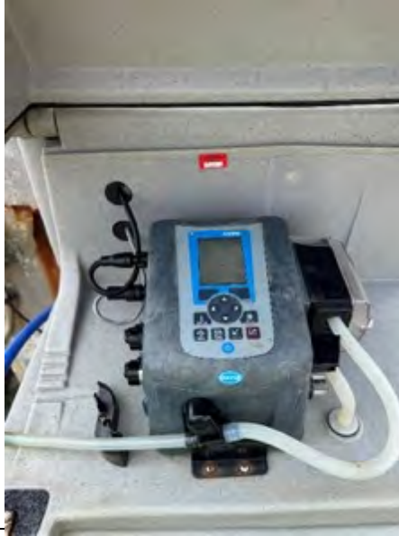
Figure 32: Effluent Sampler Control Panel
