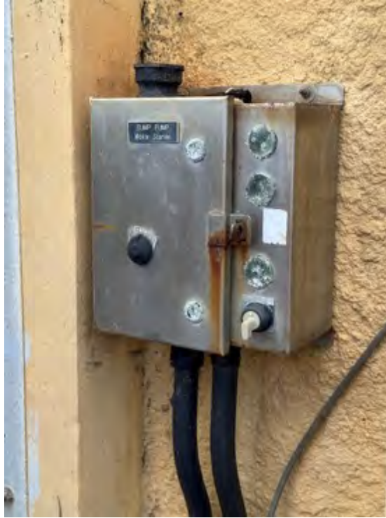
Figure 3: Dewatering Building Sump Pump Motor Starter
