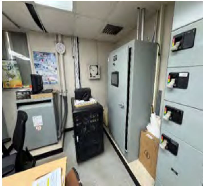
Figure 60: SCADA Server Rack
