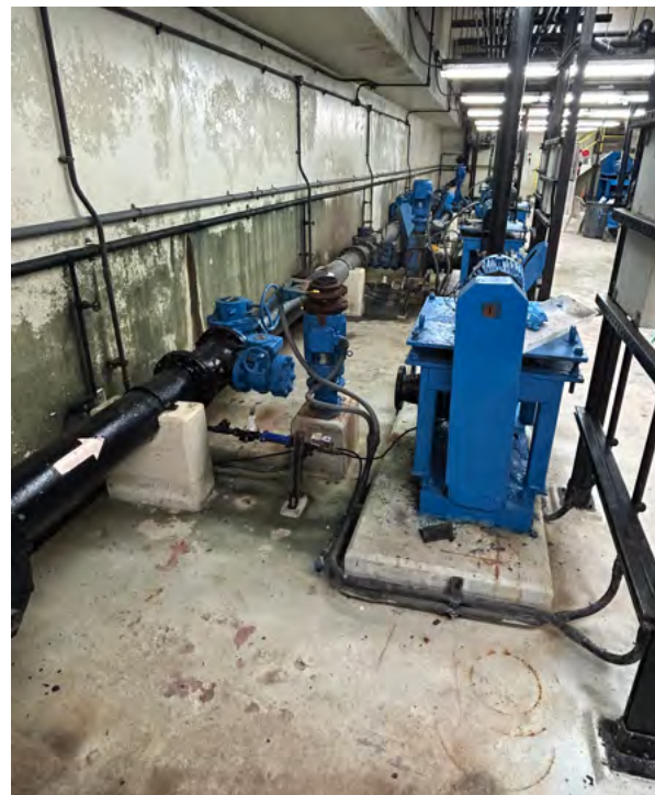
Figure 41: Primary Sludge Grinder 1 (PCTG-1) that is not installed with Primary Sludge Transfer Pump 1 (PCTP-1). The transfer pump has significant leakage.
