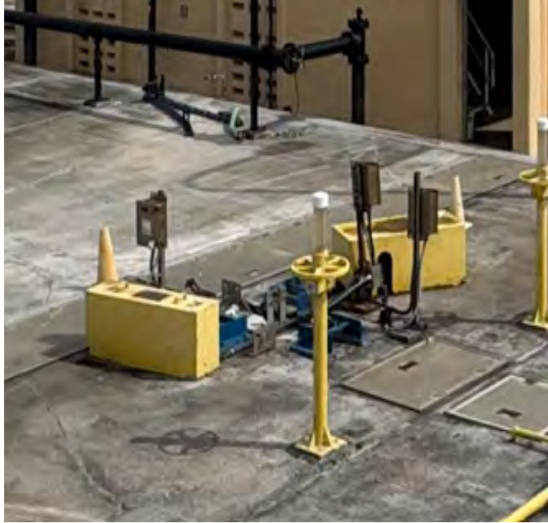
Figure 24: Clarifier 3 Cross and Longitudinal Sludge Collectors Missing
