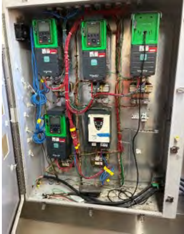
Figure 19: Flocculation Mixer VFDs
