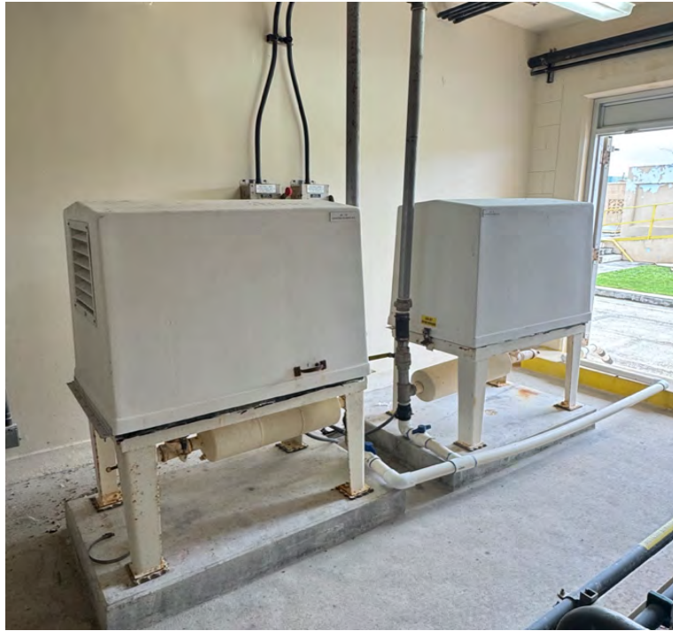
Figure 12: Aeration Blower in Chemical Room
