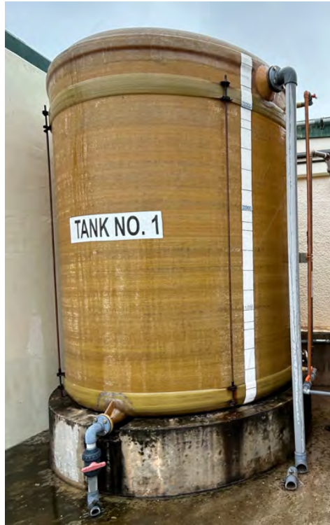
Figure 55: Chemical Day Tank 1 (Tank No. 1)
