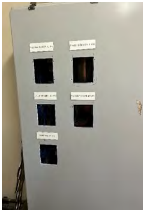
Figure 18: Flocculation Mixer VFDs Cabinet
