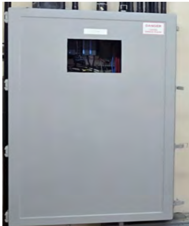
Figure 20: PLC in the Ozonation Room (PLC-OZ)
