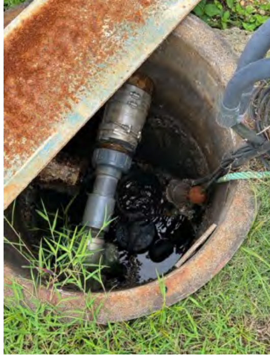
Figure 4: Operations Building Sump Pump
