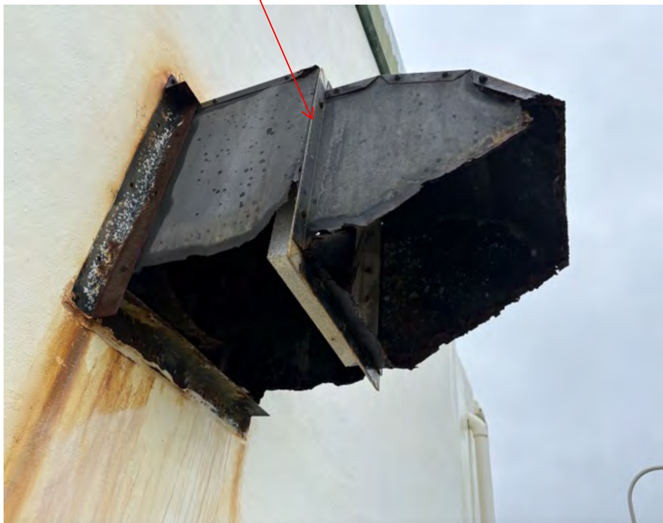
Chemical building vent
