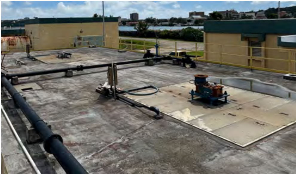
Figure 53: Aerobic Digesters with no Mixers
