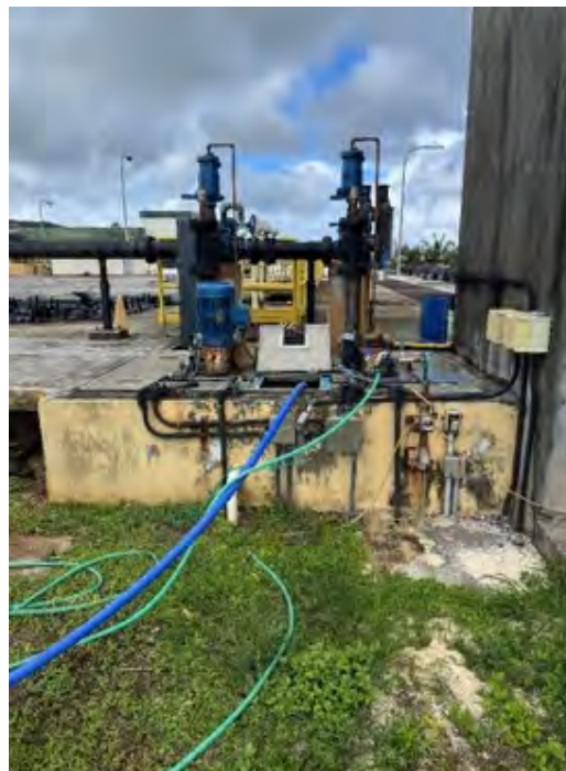
Figure 28: Primary Clarifier Scum Pump Station
