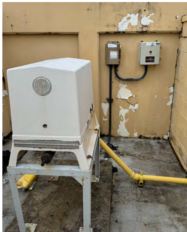
Figure 13: Aeration Blower in Solids Area.
