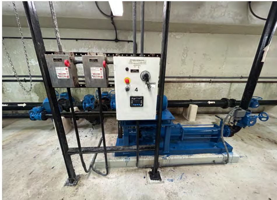
Figure 37: Primary Sludge Grinder 4 (PCTG-4) with Primary Sludge Transfer Pump 4 (PCTP-4).
