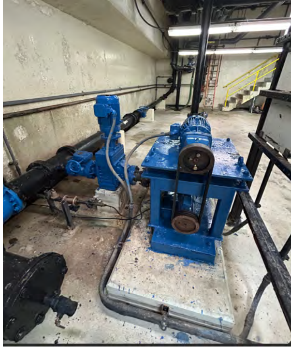
Figure 38: Primary Sludge Grinder 4 (PCTG-4) with Primary Sludge Transfer Pump 4 (PCTP-4).
