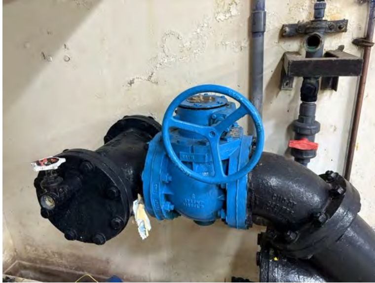
Figure 47: Digester isolation valve (ground floor)
