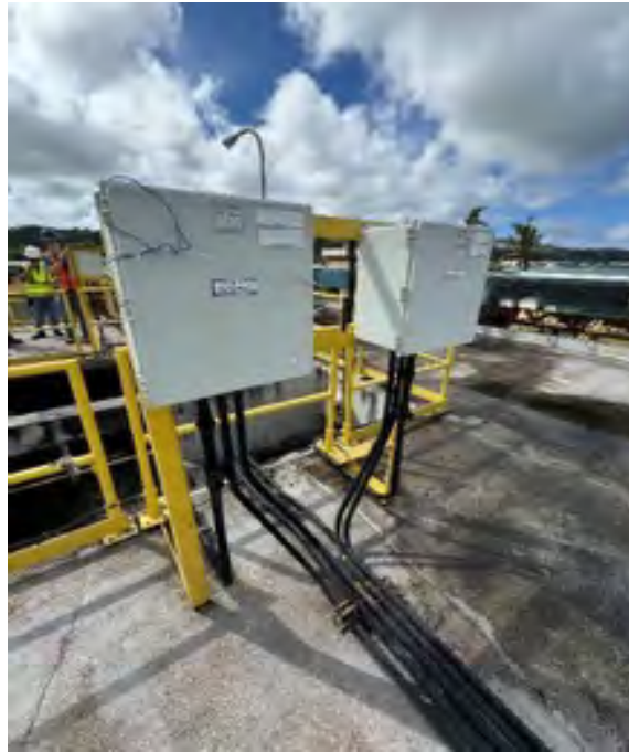
Figure 17: Flocculation Mixer Control Panels
