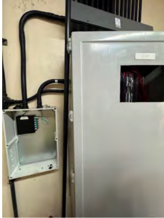
Figure 63: PLC OZ Missing OIT
