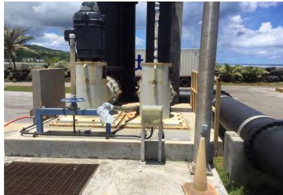
Figure 33: Effluent Pump Station
