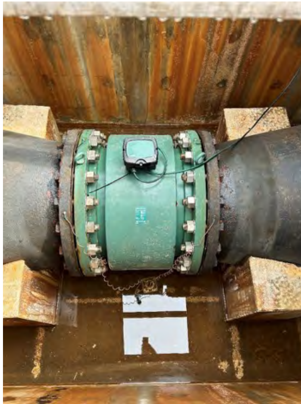
Figure 6: Influent Magnetic Flow Meter
