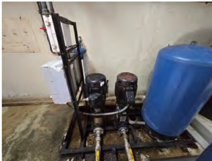
Figure 51: Booster Pump Skid
