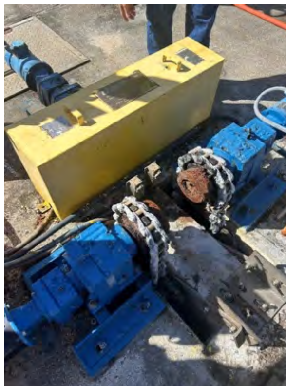
Figure 26: Longitudinal Sludge Collector Clarifier 1 (PC-2A and PC-2B)
