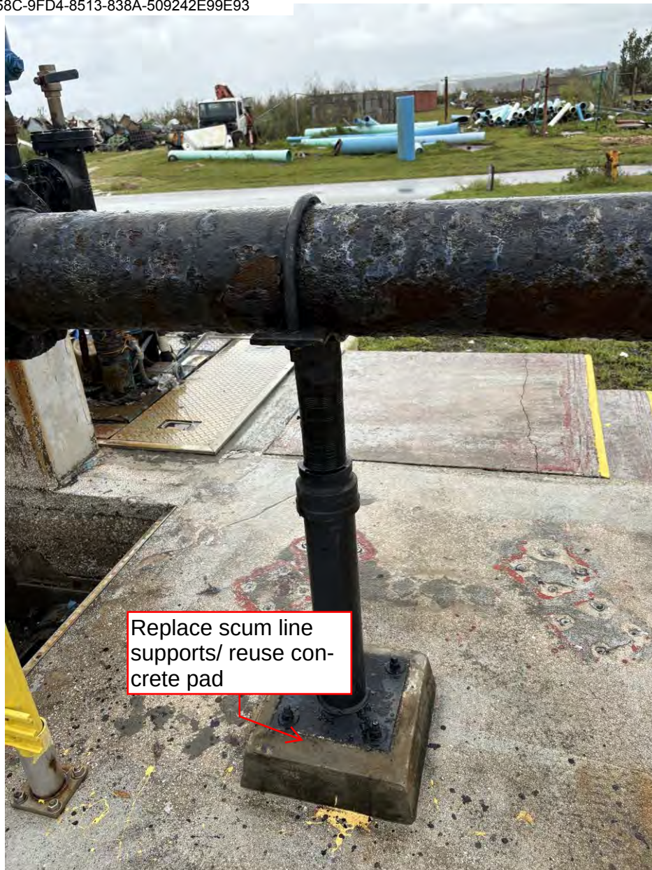
Scum pipe support
