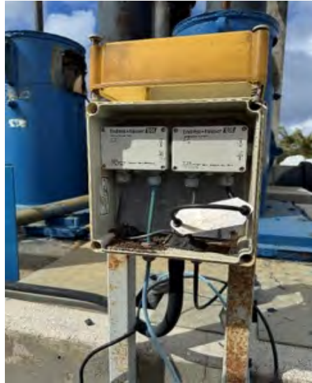
Figure 35: Level Instrument Terminal Box Enclosure
