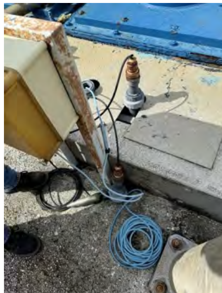
Figure 34: Two Level Instruments for the Effluent Pump Station
