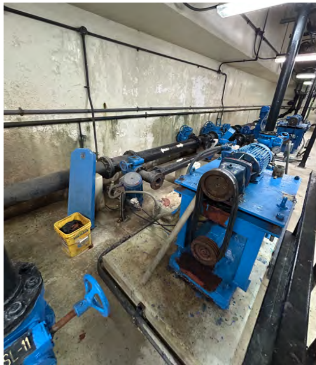
Figure 39: Primary Sludge Grinder 3 (PCTG-3) that is not installed with Primary Sludge Transfer Pump 3 (PCTP-3).
