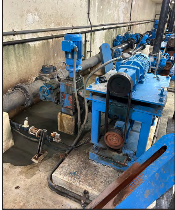
Figure 40: Primary Sludge Grinder 2 (PCTG-2) with Primary Sludge Transfer Pump 2 (PCTP-2). The transfer pump has significant leakage.
