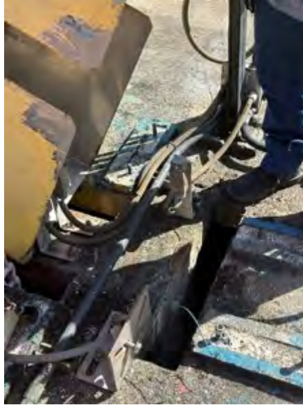
Figure 27: Missing Longitudinal Sludge Collector Clarifier 3 (PC-3A and PC-3B)
