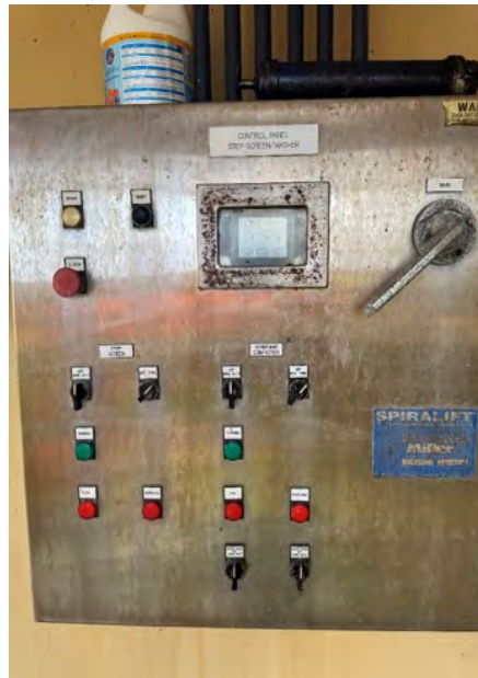
Figure 8: Step Screen Control Works Franklin Miller Control Panel
