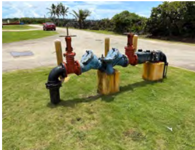
Figure 5: Water Meter and Backflow Preventer
