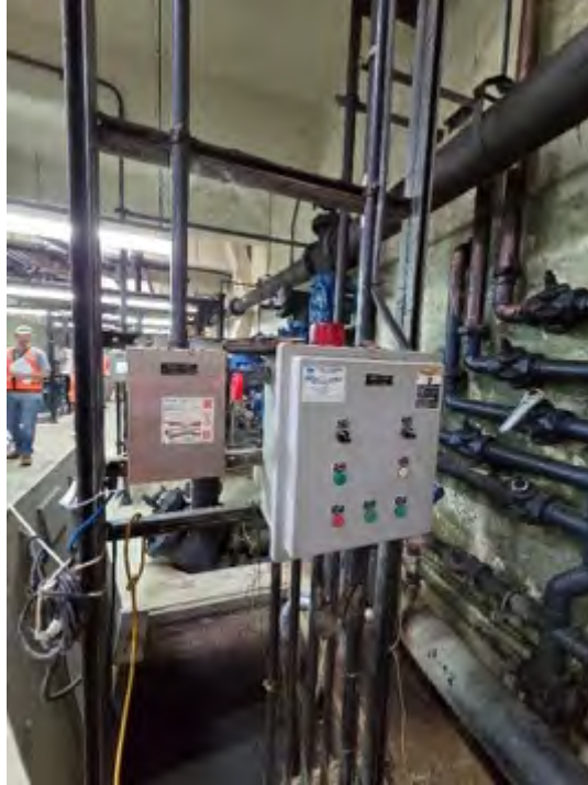
Figure 50: Pump Gallery Sump Pump Control Panel
