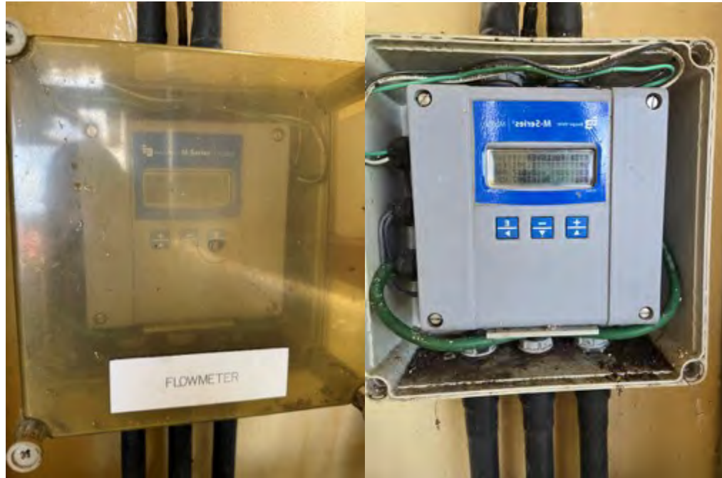
Figure 7: Influent Magnetic Flow Meter Display Unit
