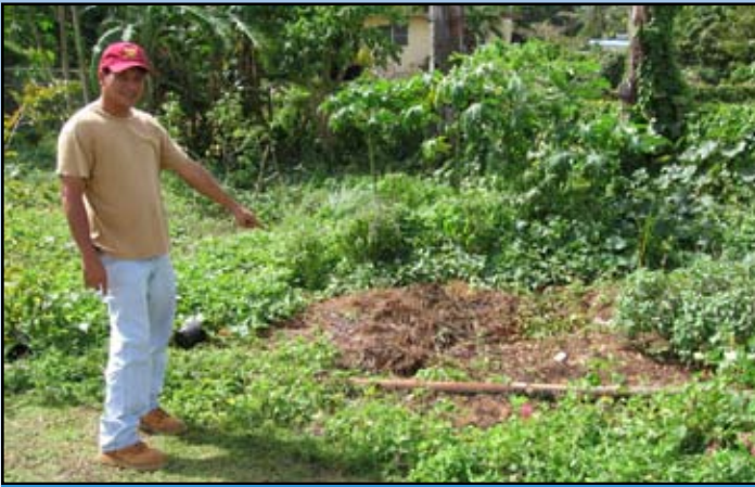
Henry pointing out an exposed four inch line in Sinajana.
